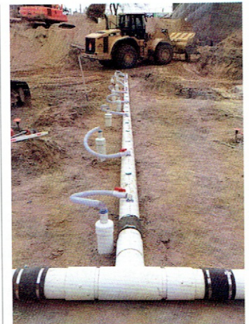
Polyvinyl chloride (PVC), mini-vacuum well-assembly installed in the borehole drilled with a track-mounted Geoprobe hollow-stem drilling rig.
