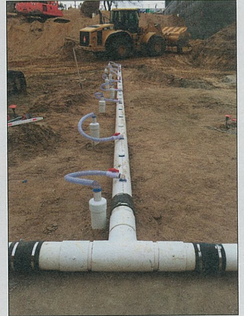
Completed installation of the PVC mini-vacuum well assembly following drilling of the borehole, utilizing track mounted Geoprobe hollow stem drilling rig.
