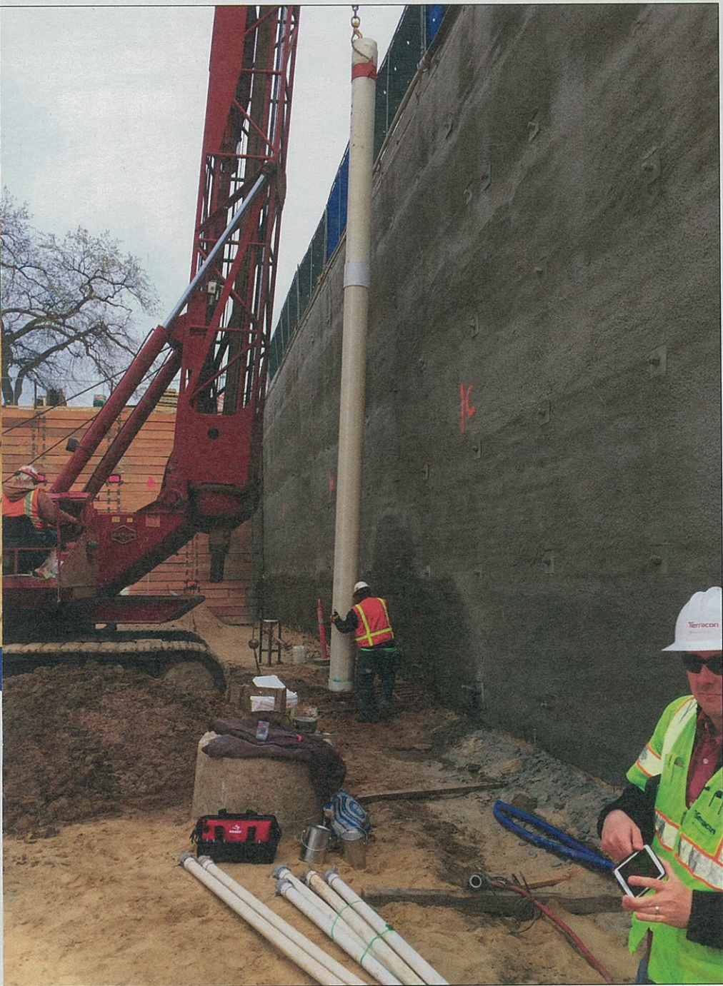
Placement of the PVC dewatering well assembly following drilling of the bore hole with the track mounted Watson drilling rig.
