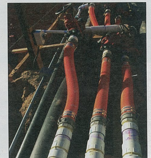
Unique, innovative groundwater collection lines allowed clean groundwater to be directed to the city storm sewer drain, contaminated-treatable groundwater to an on site groundwater treatment system, or contaminated, untreatable groundwater to be re-injected back into the ground, to its original source.
