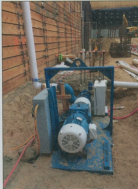
TerraFirma utilizes Holland's Rotary Lobe wellpoint pump for its mini-vacuum well dewatering system. The traditional deepwell dewatering wells can be seen in the background.
