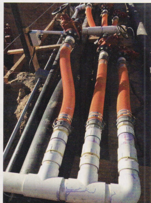
Groundwater collection lines allowed clean groundwater to be directed to the city storm sewer drain; contaminated, treatable groundwater to an onsite groundwater treatment system; and contaminated, untreatable groundwater to be re-injected into the ground, to its original source.
