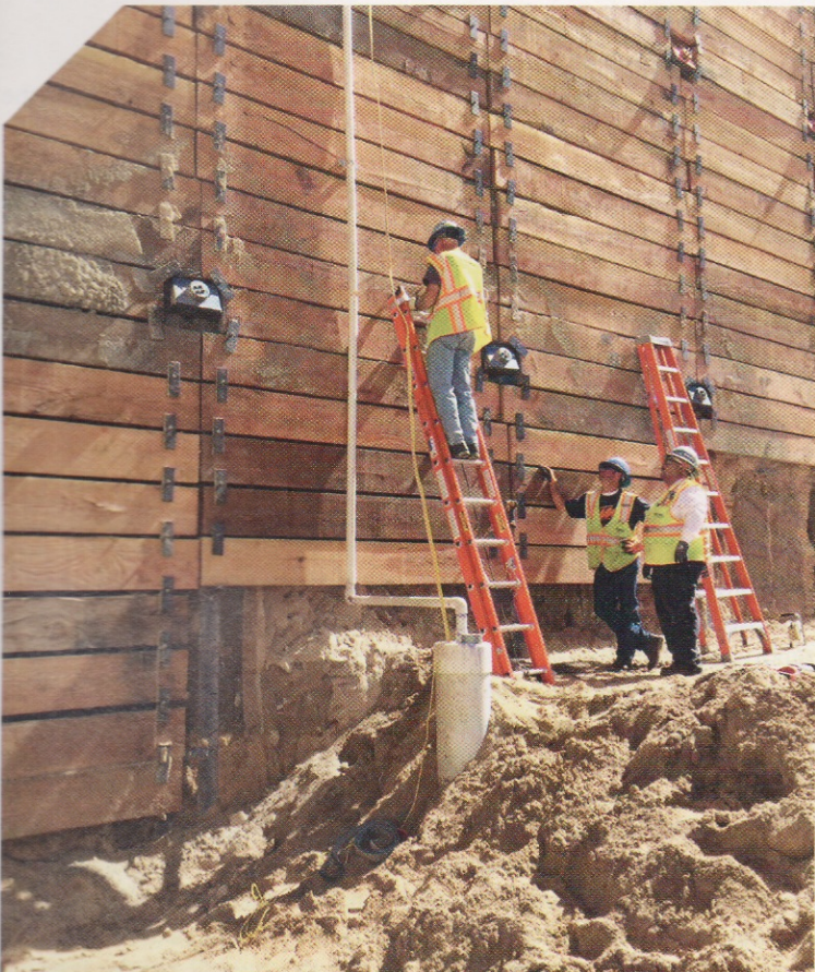
TerraFirma's well modification in progress. Wells must be lowered as excavation advances.
