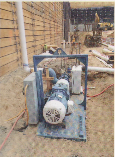
TerraFirma utilizes Holland's Rotary Lobe wellpoint pump for its mini-vacuum well-dewatering system. Traditional deep well dewatering wells are visible in the background.
