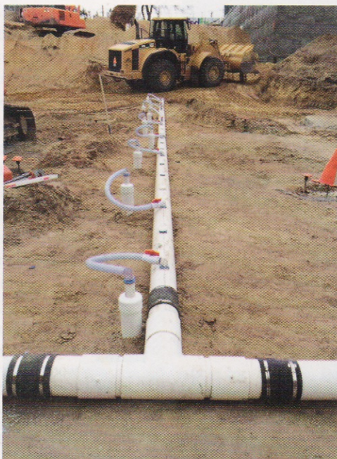
A PVC mini-vacuum well assembly was installed following drilling of the borehole using a track-mounted Geoprobe hollow stem drilling rig.
