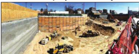
TerraFirma Earth Technologies completed dewatering of 100 Saint Paul LLC's site in Cherry Creek, where construction of a 310,000-square-foot retail and office development is underway.
